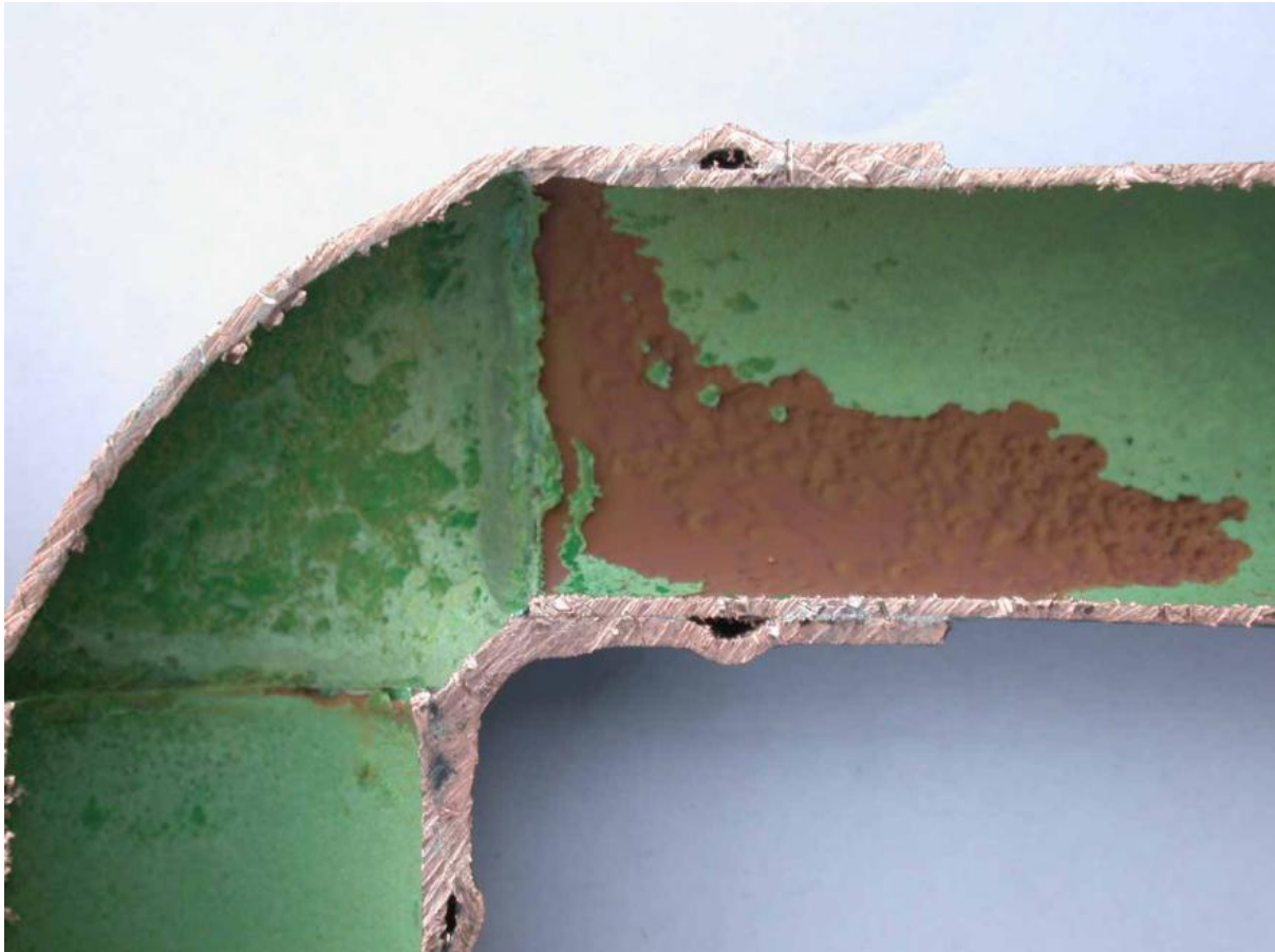
Figure 4 Erosion Corrosion at elbow.
