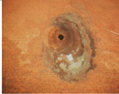
Fig. 8b – Case 15 Type 1 pitting – close up of pit
