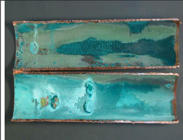
Fig. 7a – Case 4 Type 1 pitting – bore before cleaning
