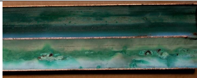
Fig. 9a – Case 23 Type 1 pitting -bore before cleaning
