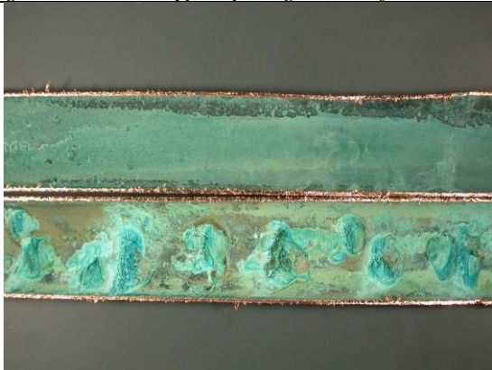
Fig. 13a – Case 3 MIC pitting -bore before cleaning
