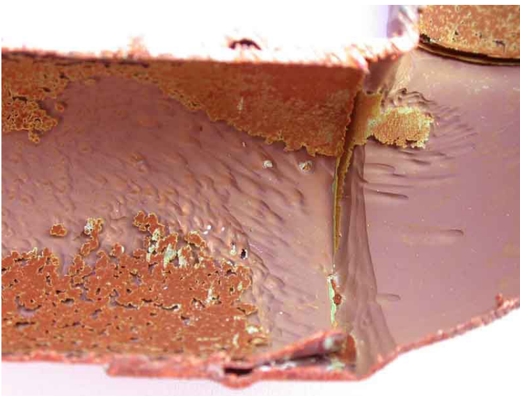
Erosion corrosion at a 22mm elbow from Slaley Hall, showing removal of protective patina on copper and grooving of copper
